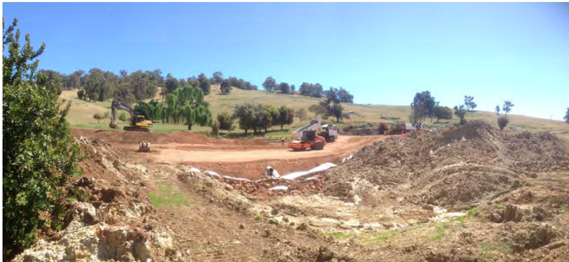
Tweed Road Failure and Corrective Works
